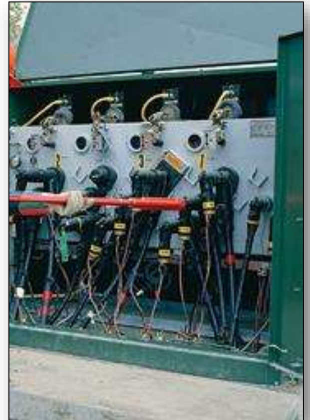
Padmount (not from actual incident)
